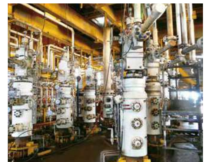
○ Five years onshore and offshore wellhead and Christmas trees project site for ptt
