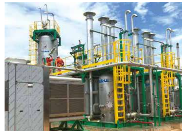
○ Ghana PSA Molecular sieve nitrogen preparation equipment working site
